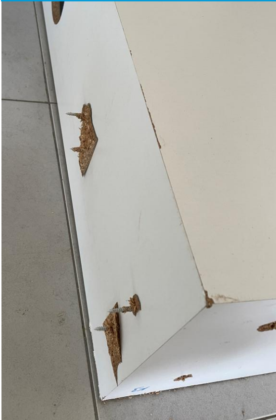
Wall elements ripped apart
